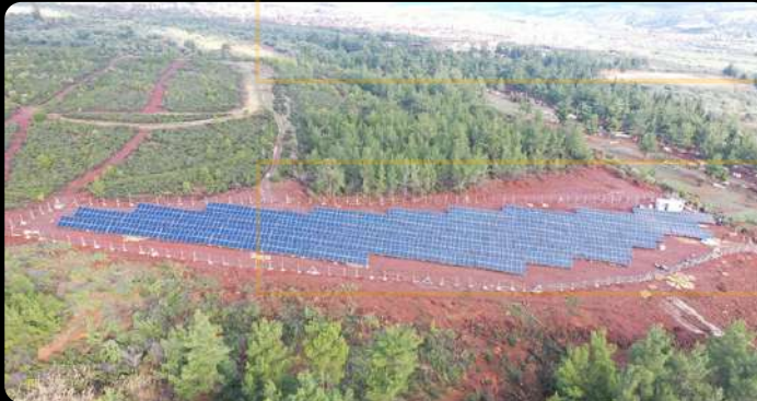
AYDIN - İLLER BANK KARACASU GES - 390KWP
